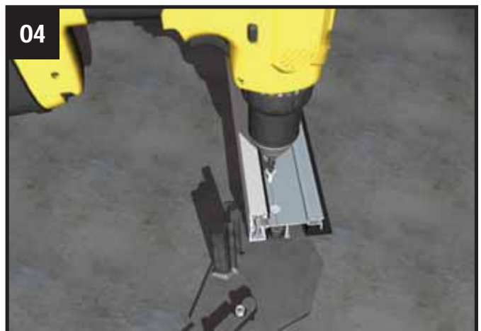
04 On the ground, away from the conservatory, offer up the first starter bar. Fasten using the set screws provided - do not over tighten.
