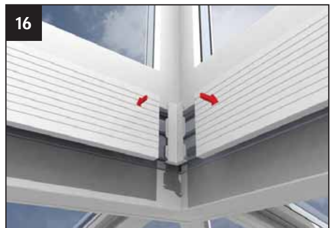
Now attach the pvc eaves beam cladding - complete the remainder of the internal claddings.
