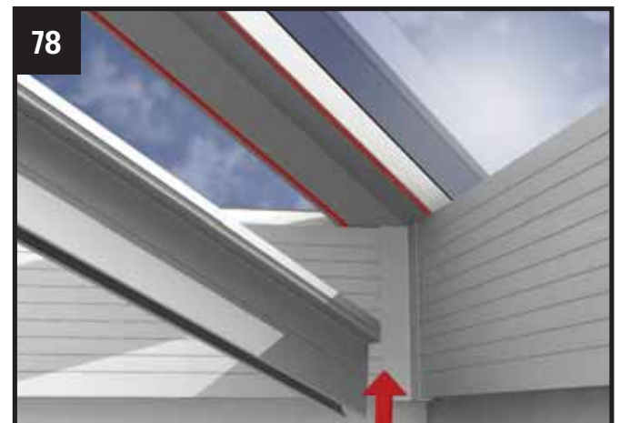
78 Complete the installation of the hip side assemblies to the Georgian bars.
