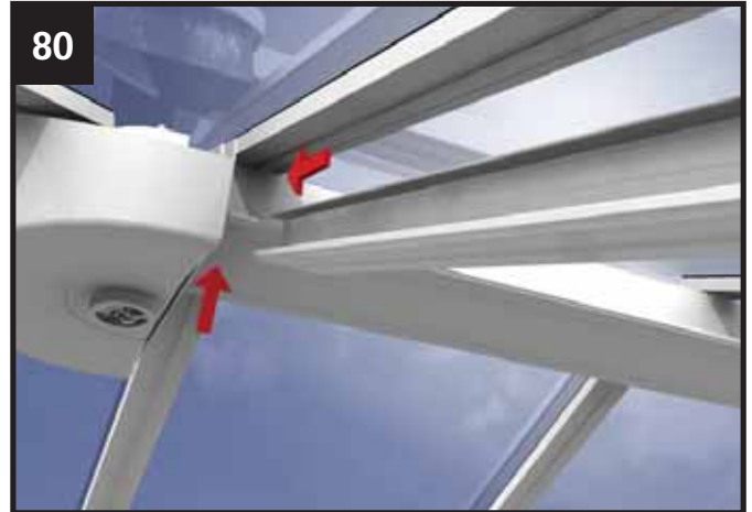
80 Attach the transom and jack rafter 'T' shaped undercladdings - always start at the ridge and work down to the eaves.
