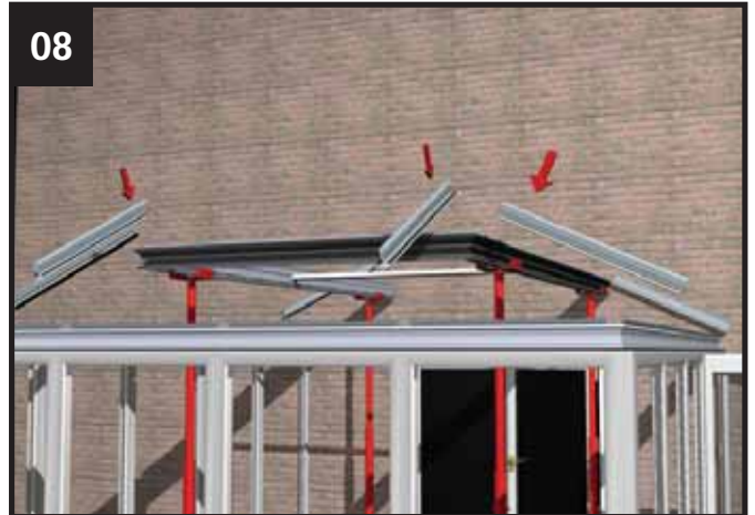
Now the Lantern eaves beam is assembled into a one piece structure, temporarily support it. Attach the glazing bars according to the component location plan. Tighten the bars, at the pagoda beam end first and then at the main eaves beam second.
