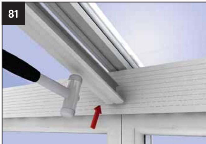
81 A plastic mallet may be necessary to tap home the 'T' shaped undercladding.
