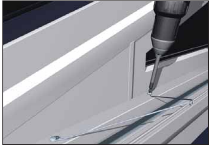
Fix wire ties at an angle as shown, ensure the Cornice is parallel to the frames/roof line.
