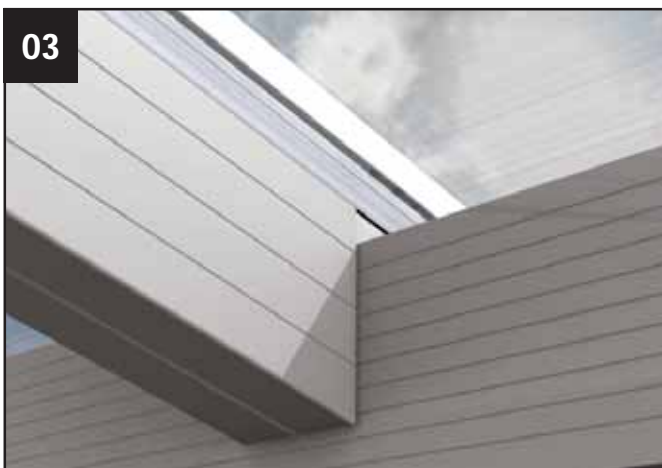
03 Measure and scribe the bolster cladding into the the eaves beam fascia board
